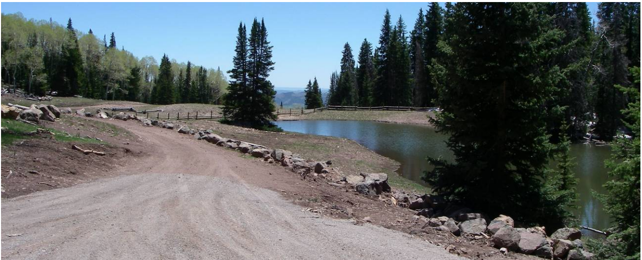
Pole fencing and rock placement along roadway to prevent OHV access to surface waters
